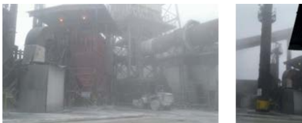
Figure 6: Rotary kiln and baghouse facility.
