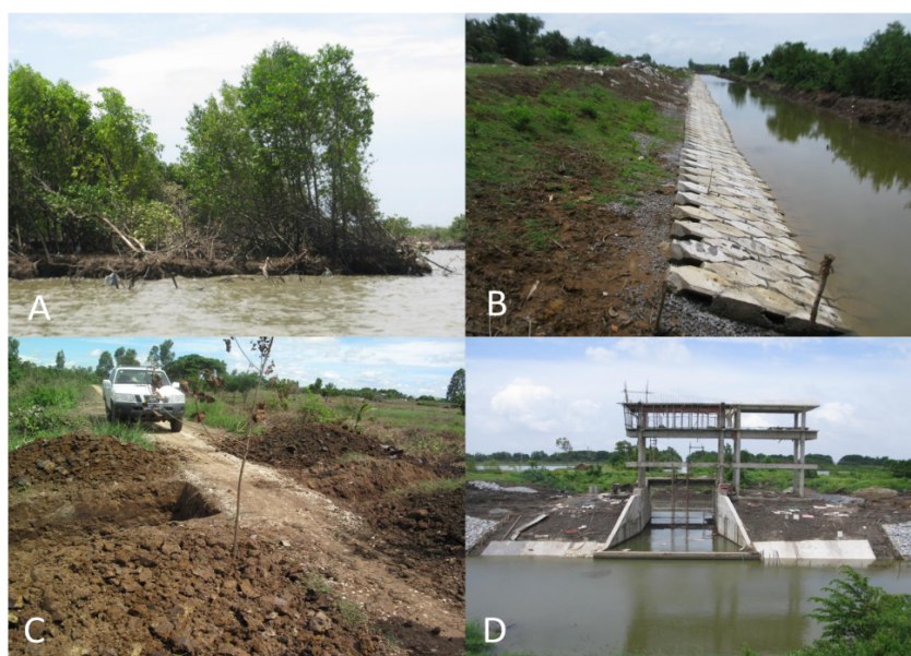
Figure 2: Status of mangroves and sea dykes in Kien Giang. (A) Mature trees of Rhizophora were uprooted; (B) Sea dykes were poorly constructed; (C) Sea dykes were damaged to install water pipes to pump saline water to aquaculture ponds located landward; (D) Newly constructed sluice gate was poorly protected and highly exposed to erosion.
