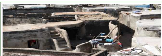
Figure 5: Indigenous staircase without a hand rail.
