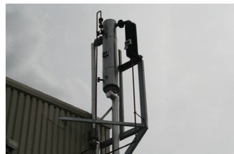
Figure 2: A picture of a light-ends removal kit installed to help improve the safety of a manufacturing plant.
