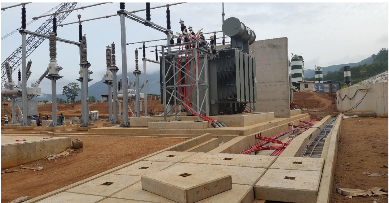
Fig. 6 Electrical Installations at the Kashimbilla Multipurpose dam
